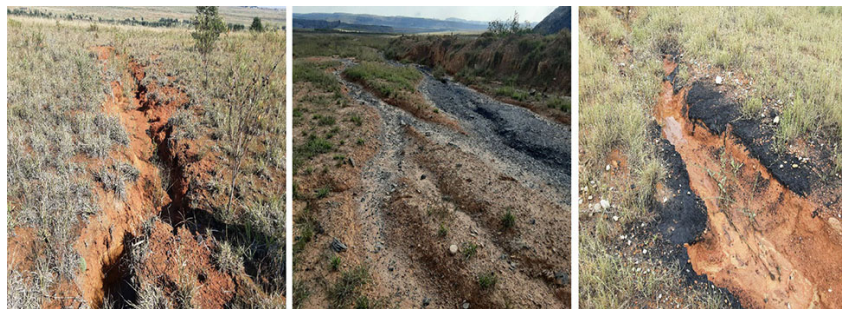
Figure 11—Severely eroded areas that require immediate intervention
