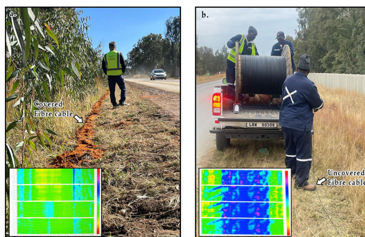
Figure 3—Deployment of distributed acoustic sensing (DAS) fibre optic cable along the nodal system profiles. (a) Insert shows the recorded signal from the covered fibre optic cable with soil and the signal is less noisy (b) Shows the uncovered fibre optic cable
