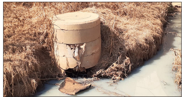
Figure 1. Vandalized sewer manhole in the study area
