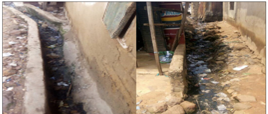
Figure 6: Unsanitary conditions of open drains in Kabawa community
