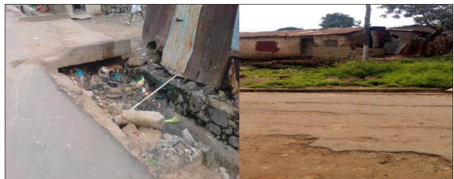
Figure 4: A bare ground covered with roofing sheets used as a bathroom with waste water channelled into the open drains in Kabawa community
