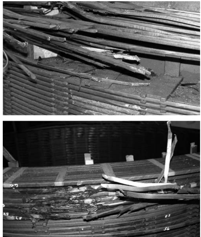
Fig. 2. Windings of Eskom transformers presumed damaged by the geomagnetic storm on 29 October 2003.
