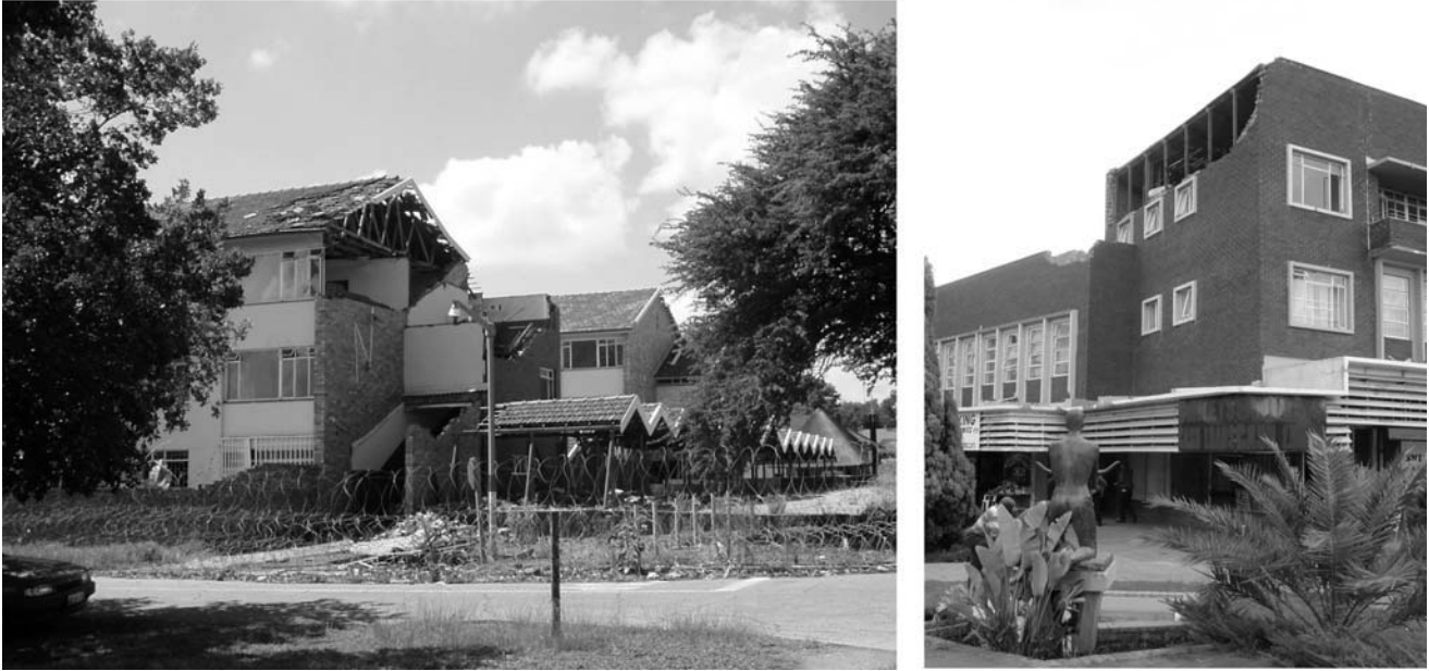
Fig. 5. Damage in Stilfontein caused by the M_L = 5.3 tremor on 9 March 2005.
