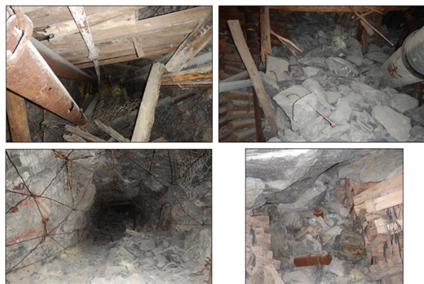
Figure 14—Compromised accessways along investigation routes
