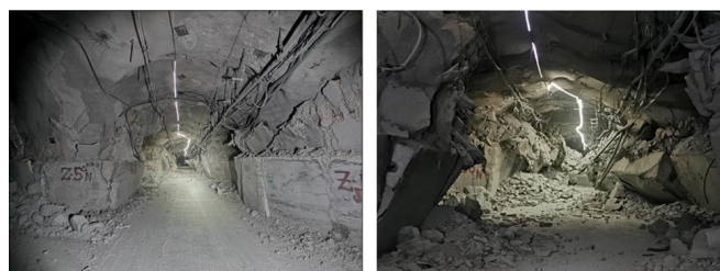
Figure 3—Damage on the production level, showing moderate damage (left) and collapse conditions (right) (images courtesy Codelco)
