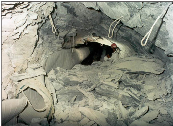
Figure 3—Examples of seismic damage to underground excavations (photograph by W.D. Ortlepp)
