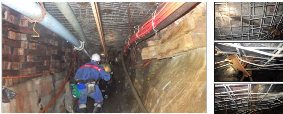
Figure 15—Protruding rockbolts and bolts installed at an acute angle
