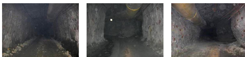
Figure 2—Variations in squeezing severity in three locations less than 100 m apart at 2150 m depth at the LaRonde Mine (Mercier-Langevin and Hadjigeorgiou, 2011)
