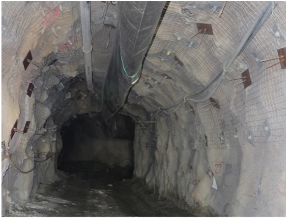
Figure 8—Use of long reinforcement to control large deformations in a hard rock mine
