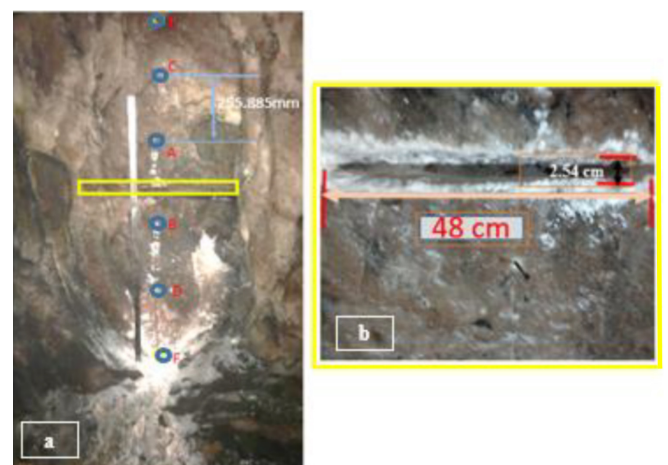
Figure 8—(a) Marking and installing the measuring points, (b) cutting of slot and its dimensions
