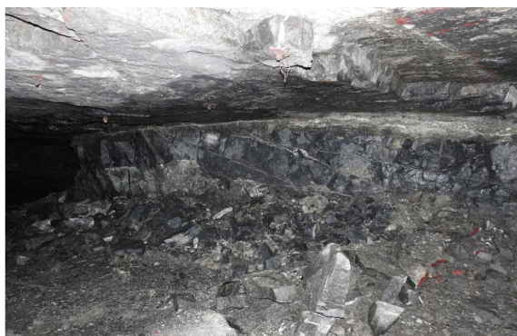
Figure 3—Failure of a pillar facilitated by the alteration zone and the presence of subhorizontal jointing in the level 2 failure zone
