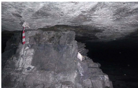
Figure 5—A pillar in the level 3 failure zone. The original size of the pillar is clearly indicated by the change in colour on the hangingwall
