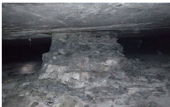
Figure 4—A pillar in the level 3 failure zone illustrating extensive scaling and failure. The core of this pillar is deemed to be still intact
