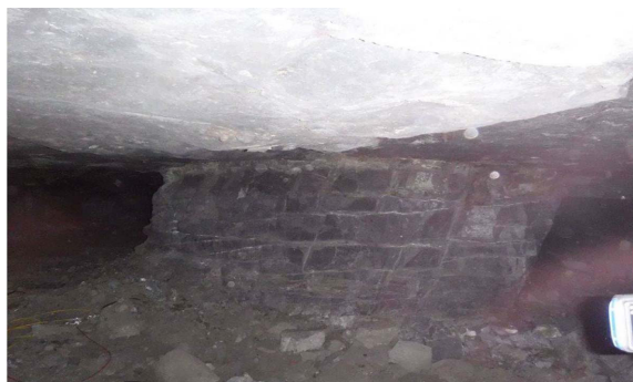
Figure 2—A pillar in the level 2 failure zone with horizontal joints and vertical tensile cracks visible
