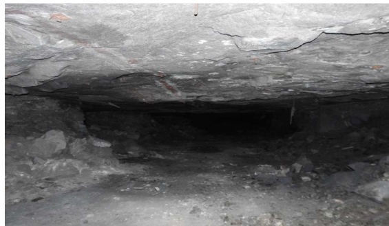
Figure 6—Pillar condition in the level 4 failure zone. The pillars are crushed, but some contact with the hangingwall is still maintained. The large spans indicate that the pillars were not cut to the planned design
