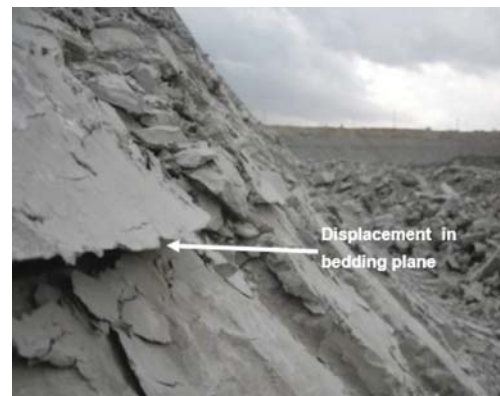
Figure 21—Movement observed in one of the major bedding planes. Horizontal displacements of up to 30 mm were noted and corroborated to deformations within perimetral inclinometers
