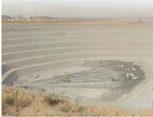
Figure 7—Condition of pit in 2007. The base level -55m AOD is dark in colour, showing the moist condition of the intact marls when first exposed
