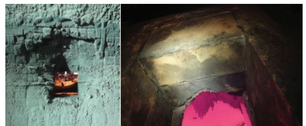
Figure 6— (Left) Endwall refractory wear in the vicinity of the tapblock observed at the time of refractory relining. (Right) Photograph through the rear copper tapblock, view angled upwards, showing the hot face wear on the lower-front extension bricks above the tap-hole. Evidence of this wear suggested that the bell-mouth funnel extended all the way back from the front of the refractory to the extension bricks; some 400 mm
