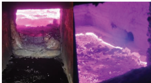
Figure 5— (Left) View of slag tap-hole hot face wear profile. Bell-mouth size estimated to be 650 x 400 mm. (Right) Photo through the rear copper tapblock from outside the furnace showing the loss of bricks in front of the tap-hole and the deterioration of the tapping bricks in the back block
