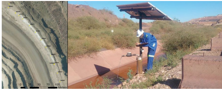
Figure 19—Location of solar powered depressurization holes with discharge into lined stormwater canal
