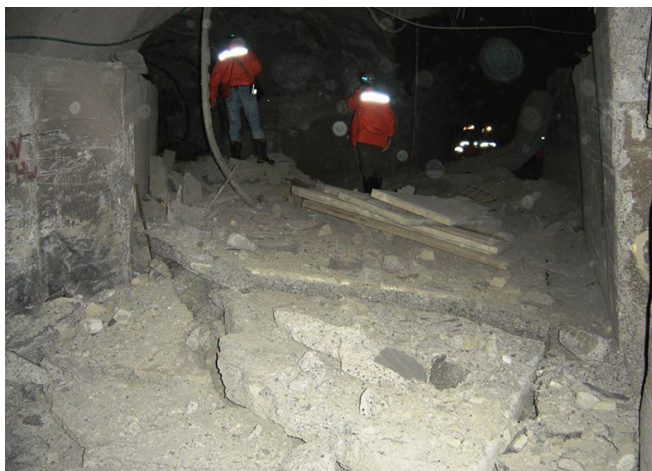
Figure 3—Concrete floor heave of nearly 2 m caused by a rockburst (Stacey and Rojas, 2013; photograph T.R. Stacey)
