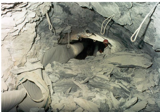
Figure 2—Rockburst damage and fragmentation (Stacey and Rojas, 2013; photograph W.D. Ortlepp)
