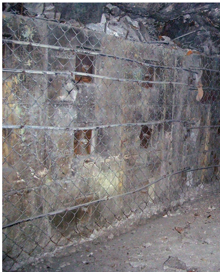
Figure 6—Remedial 'staple' support with wire ropes (Stacey and Rojas, 2013; photograph Y. Potvin)
