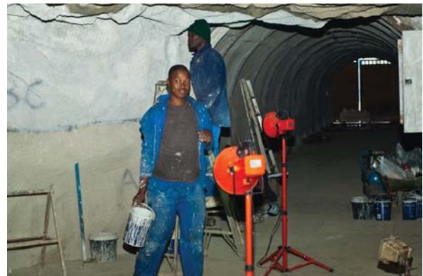
Figure 2—Moulding the tunnel wall to simulate exposed rock face in the Wits Mine Tunnel (2013)
