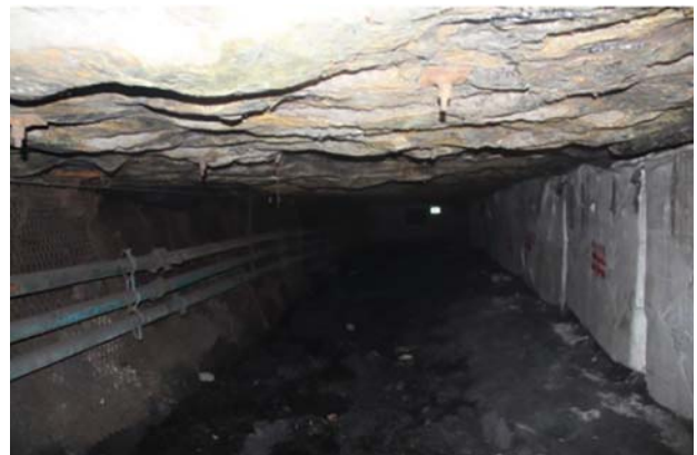
Figure 16—Photograph of the entry retention effect
