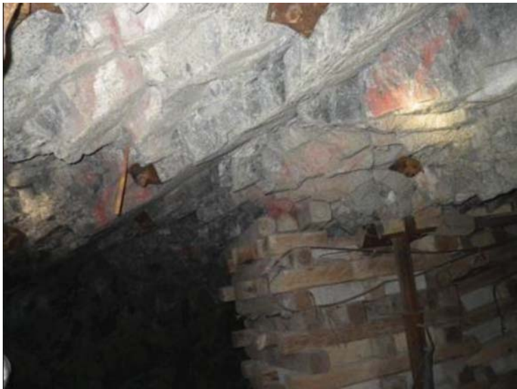
Figure 19—Condition of the quartzite hangingwall, where the bedding planes were exposed in the back area of the LI25-23 Libanon Reef stope
