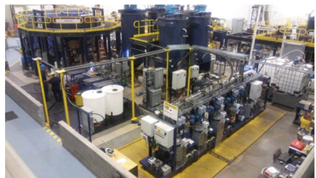
Figure 6—FLSmidth's pilot plant facility under construction in the technology centre in Salt Lake City, USA
