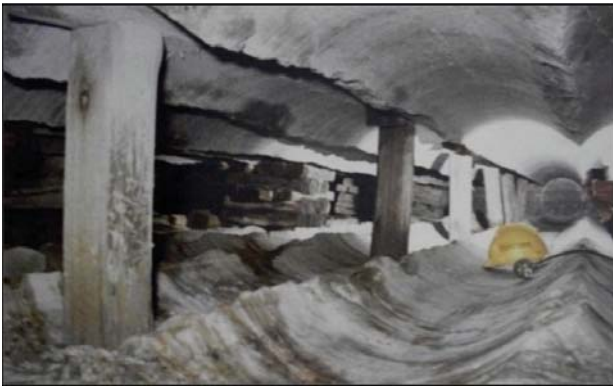
Figure 1—The completed slot bored by sequential raisebore holes at West Driefontein (Adams, 1978)
