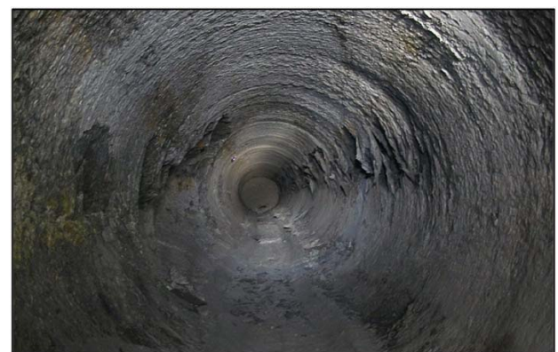
Figure 15—Photograph of hole 17 taken from the upper reef drive, showing spalling on the western (right) sidewall that occurred only after the hole 18 was drilled
