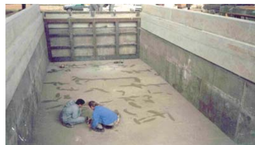
Figure 4—Surface tearing of a potassium silicate concrete floor
