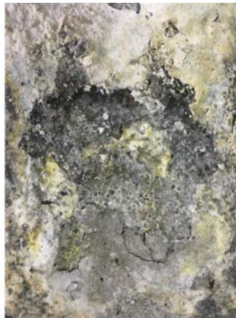
Figure 5—Surface scaling of acid-resistant concrete in wet/dry sulphuric acid conditions
