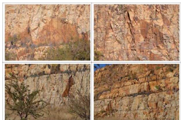
Figure 12—Closer views in the southerly direction of the smooth wall blasted N4 road cutting, in which some wedge failures are visible
