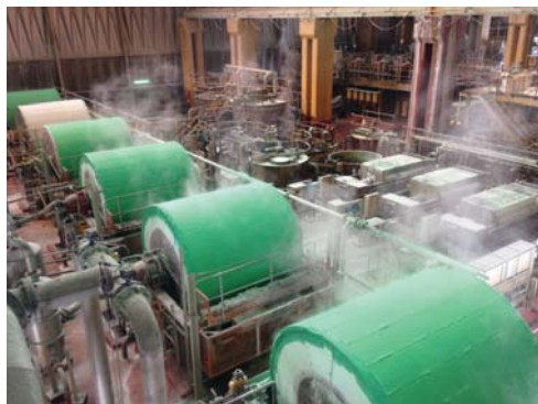
Figure 3—Photograph of the sulphur removal section showing the rotary vacuum drum filters in the foreground and the polishing filters, precipitation, and dissolution reactors in the background
