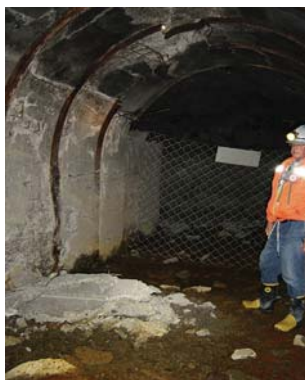
Figure 6—Rockburst damage caused by floor heave (Stacey and Rojas, 2013)
