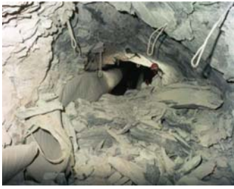
Figure 1 – Rockburst damage and fragmentation (Stacey and Rojas, 2013)
