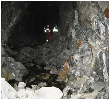
Figure 5—Rockburst damage in lower sidewalls of tunnel (Stacey and Rojas, 2013)
