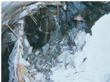
Figure 2 – Protruding rock support elements after dynamic (rockburst) rock failure (Stacey and Rojas, 2013)
