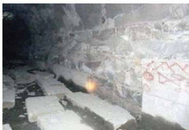
Figure 7—Concrete support panels ejected during a rockburst event (Stacey and Rojas, 2013)
