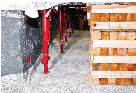
View looking up-dip showing the edge of the gully, mechanical props, and gully pack
