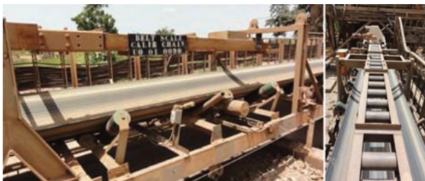
Figure 10—Calibration of the plant feed weightometer using (a) the zero test, and (b) a static weight test
