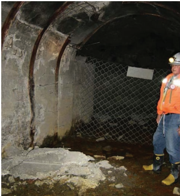
Figure 7—Rockburst damage caused by floor heave (photograph T.R. Stacey)
