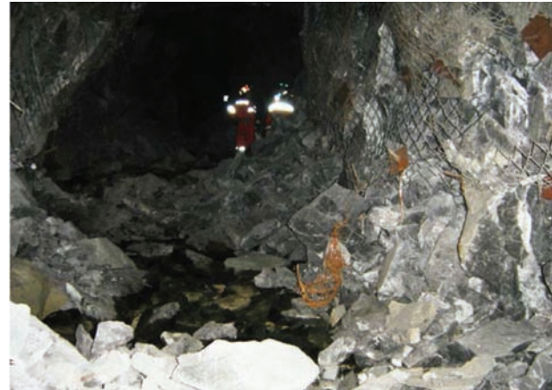
Figure 8—Rockburst damage in lower sidewalls of tunnel (photograph T.R. Stacey)
