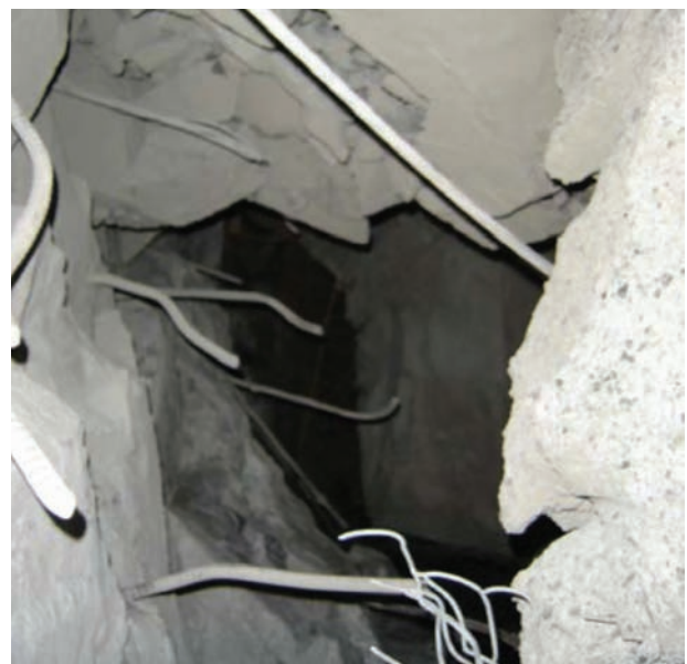
Figure 10—Broken rockbolts and cables behind concrete wall (photograph T.R. Stacey)
