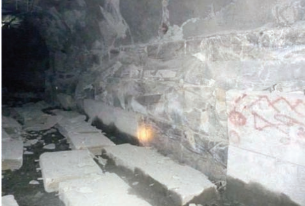
Figure 11—Concrete support panels ejected during a rockburst event (photograph Y. Potvin)
