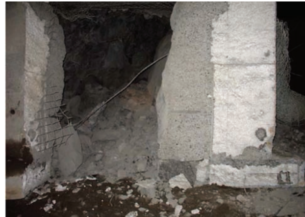
Figure 9—Lateral movement of concrete wall (photograph T.R. Stacey)
