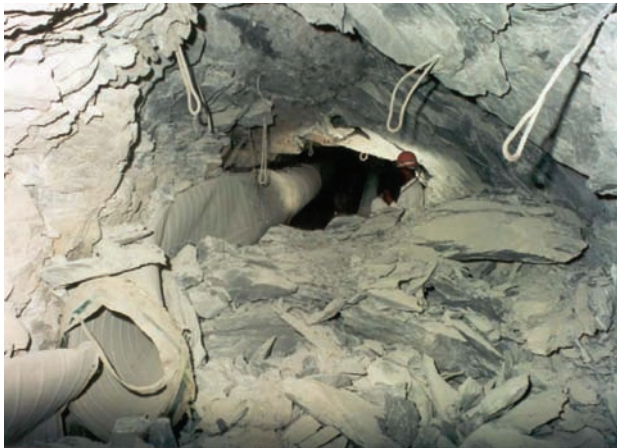
Figure 1—Rockburst damage and fragmentation (photograph W.D. Ortlepp)
