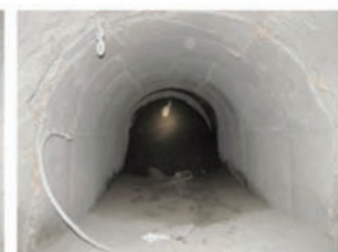
(e) Mud in back of Drift 13 near RAW
