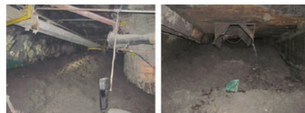
(a) Mud in rim tunnel at Drift 10
