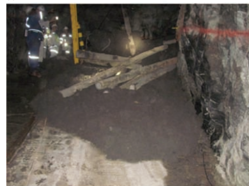
(c) Mud in access ramp into western end at Drift 15
