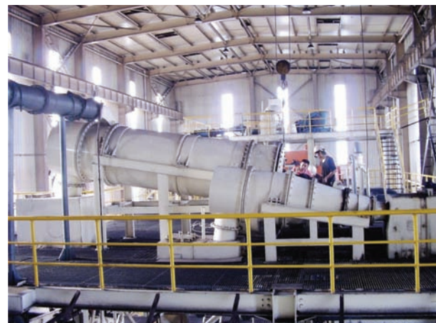
Figure 6 – Three-product cyclone installation in China
