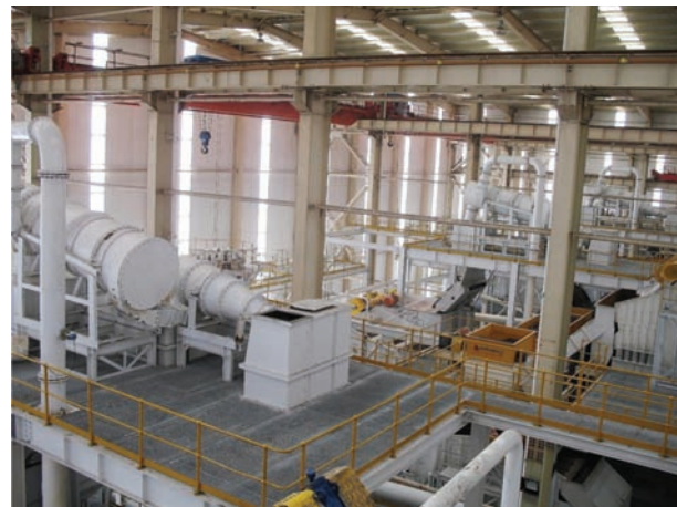
Figure 5 – Three-product cyclone installation in China
