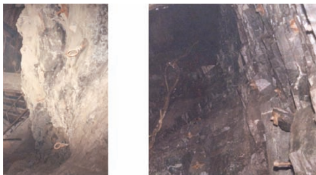
Figure 1—Structural failures in orepasses
