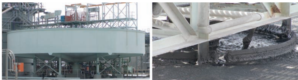
Figure 14—P266E feedwell installed in a 16.5 m diameter platinum concentrate thickener at Anglo American Platinum's Western Limb Tailings Retreatment Plant (photos courtesy of Anglo American Platinum)
