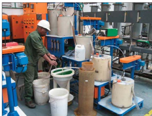
Figure 5b—The integrated plant's neutralization reactors, comprising a feed tank (hidden) and five 20-litre reactors arranged in series; in the foreground are various settlers that were used during the operation of this plant
