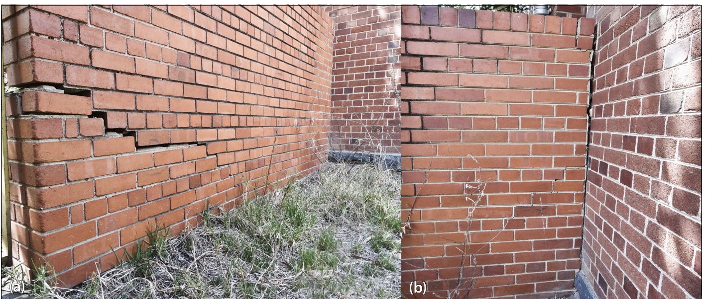
Figure 4 A later additional wall showing typical damage due to soil movement
