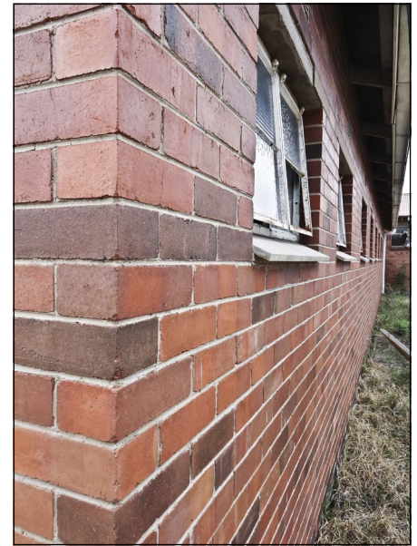
Figure 3 Closer view of the outside wall of one of the abandoned buildings
