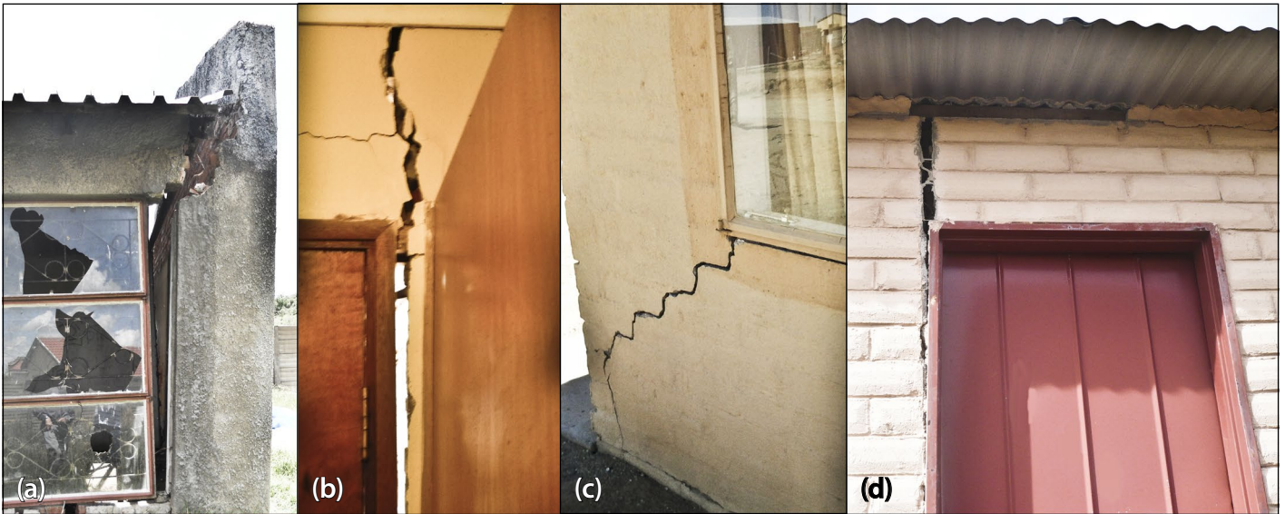
Figure 5 Four single-storey masonry houses failing within a few years after construction
