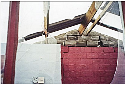
Figure 1 Damage of gable wall and failure of a roof caused by inadequate roof anchorage (Goliger 2002 – permission for re-use of photo granted)
