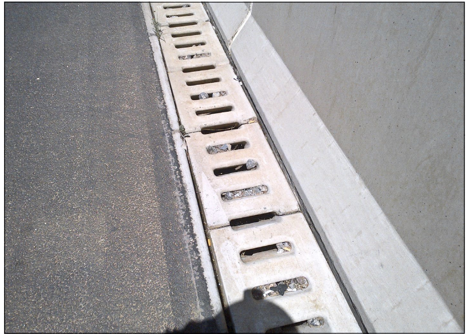
Figure 1 Clogging of slotted inlets
