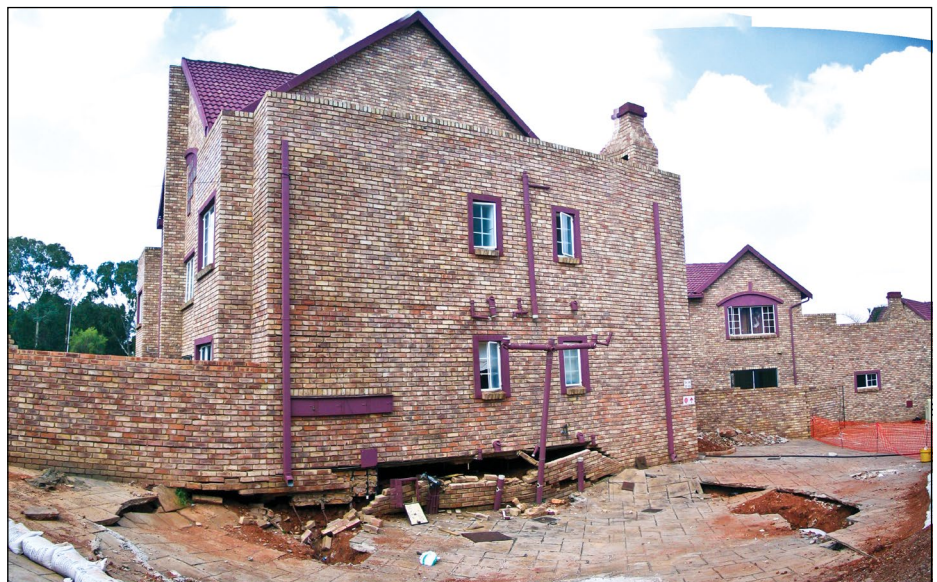
Figure 10 Two-storey residential building structurally damaged by 15 m sinkhole
