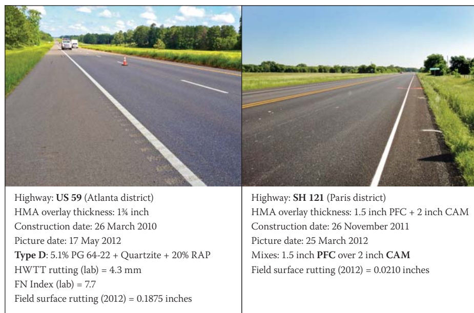
Figure 8 Field rutting performance of US 59 and SH 121 highways
