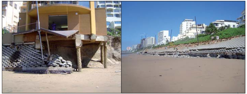
Figure 5 Failure of loffelstein seawall at Umhlanga main beach (eThekweni Municipality database, March 2007)
