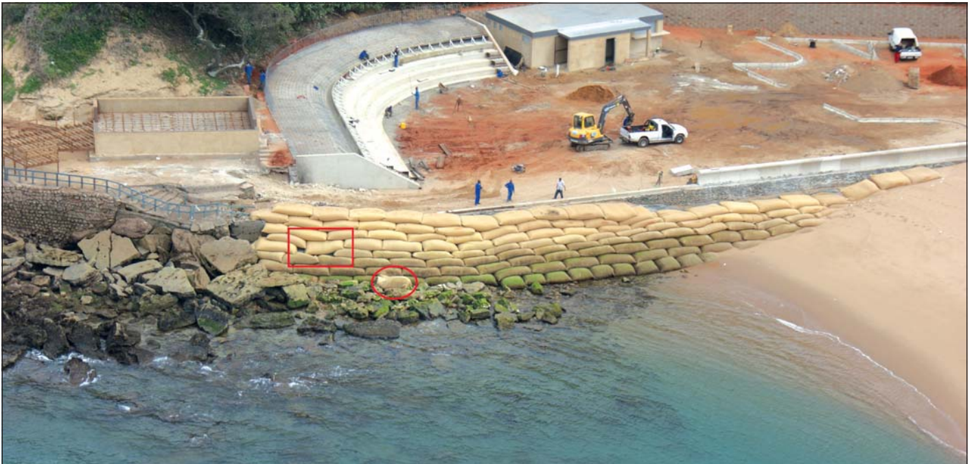
Figure 10 A geotextile bag wall failure at Isipingo (July 2011). The red rectangle highlights where a bag was removed from the wall and the red circle identifies the removed bag
