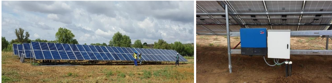
Figure 4: View of 75 kWp solar plant at the aquaculture centre, and one of the inverters.
