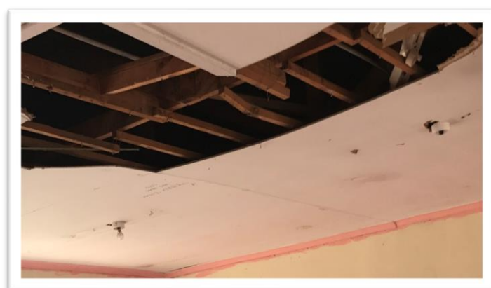
Image 2: Collapsing Roof: Gede Primary
