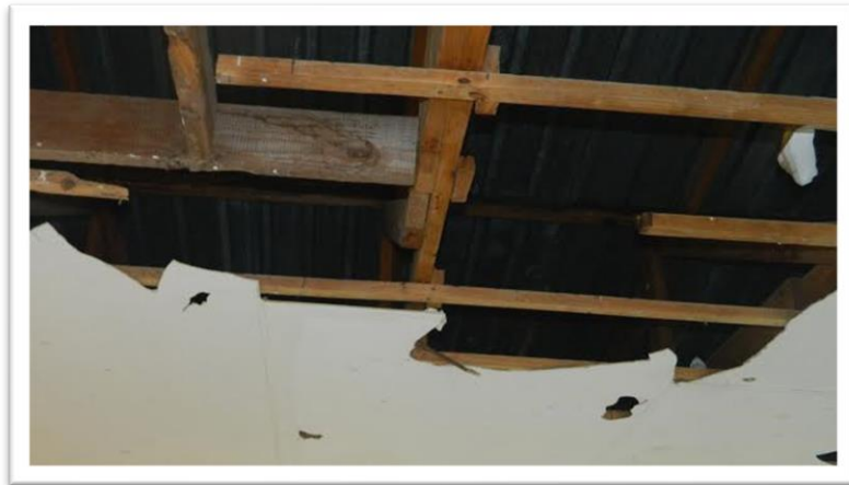
Image 3: Collapsing Roof: Rivoningo Primary
