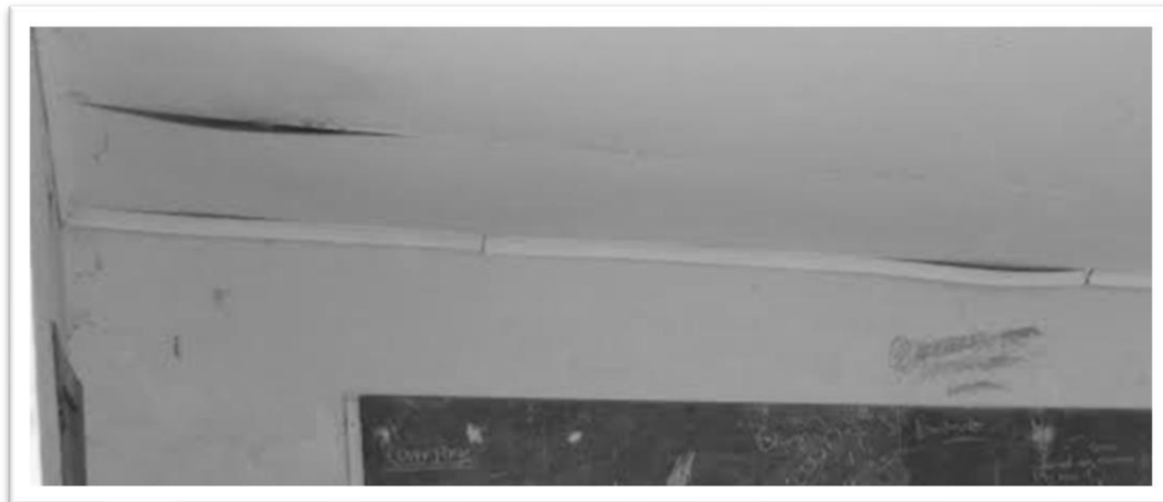
Image 4: Collapsing Ceiling: Tlanga Primary
