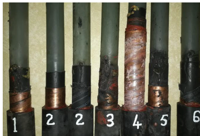
Fig. 8. Cable terminations after all accessories have been removed to reveal the root cause failure
