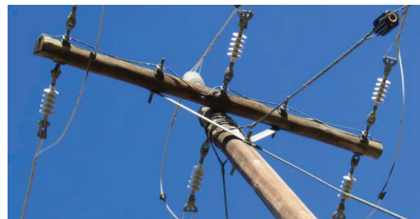
Fig. 15 The stay wires reduce the BIL of the line at strainer poles.
