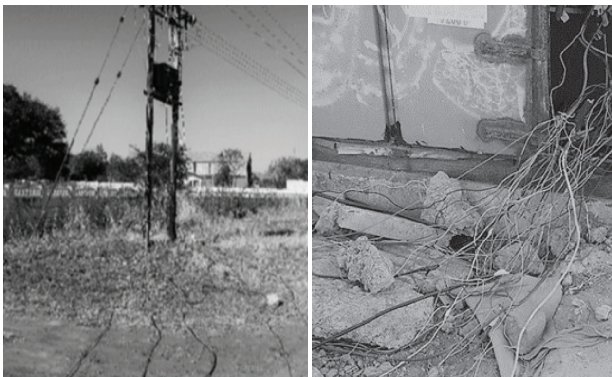
Fig. 1: Left: Illegal connection. Right: Live wires illegally connected to supply and lying on the ground [16], [19]
